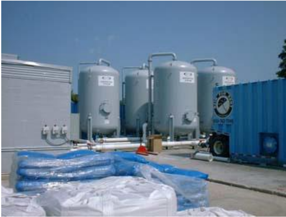
Onsite water treatment plant, Upper Sheboygan River, 2007
